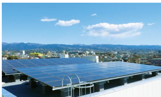
Solar power generation system installed at the Fuji Plant
